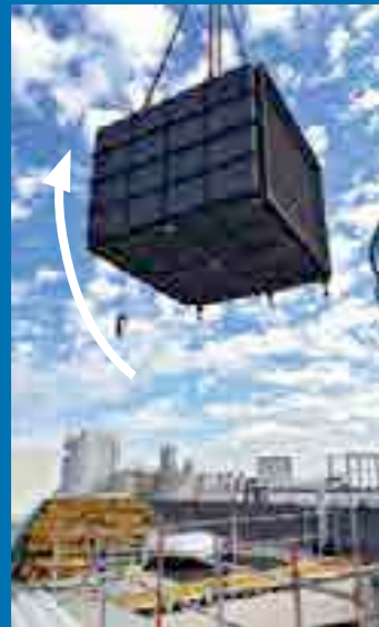
The old tank (top) is replaced with a new gas economizer (bottom) to recover heat more efficiently.
